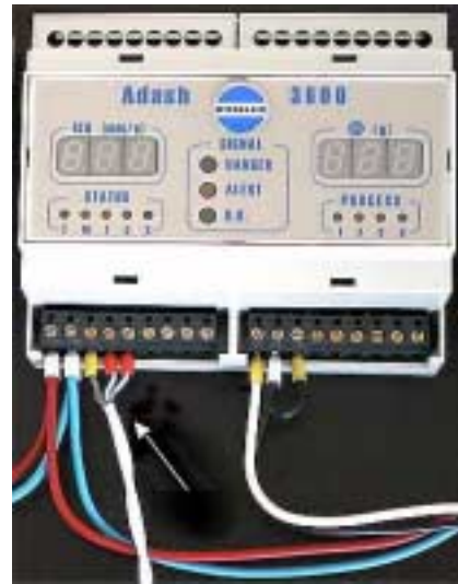
Fig. Connection of the vibration sensor
